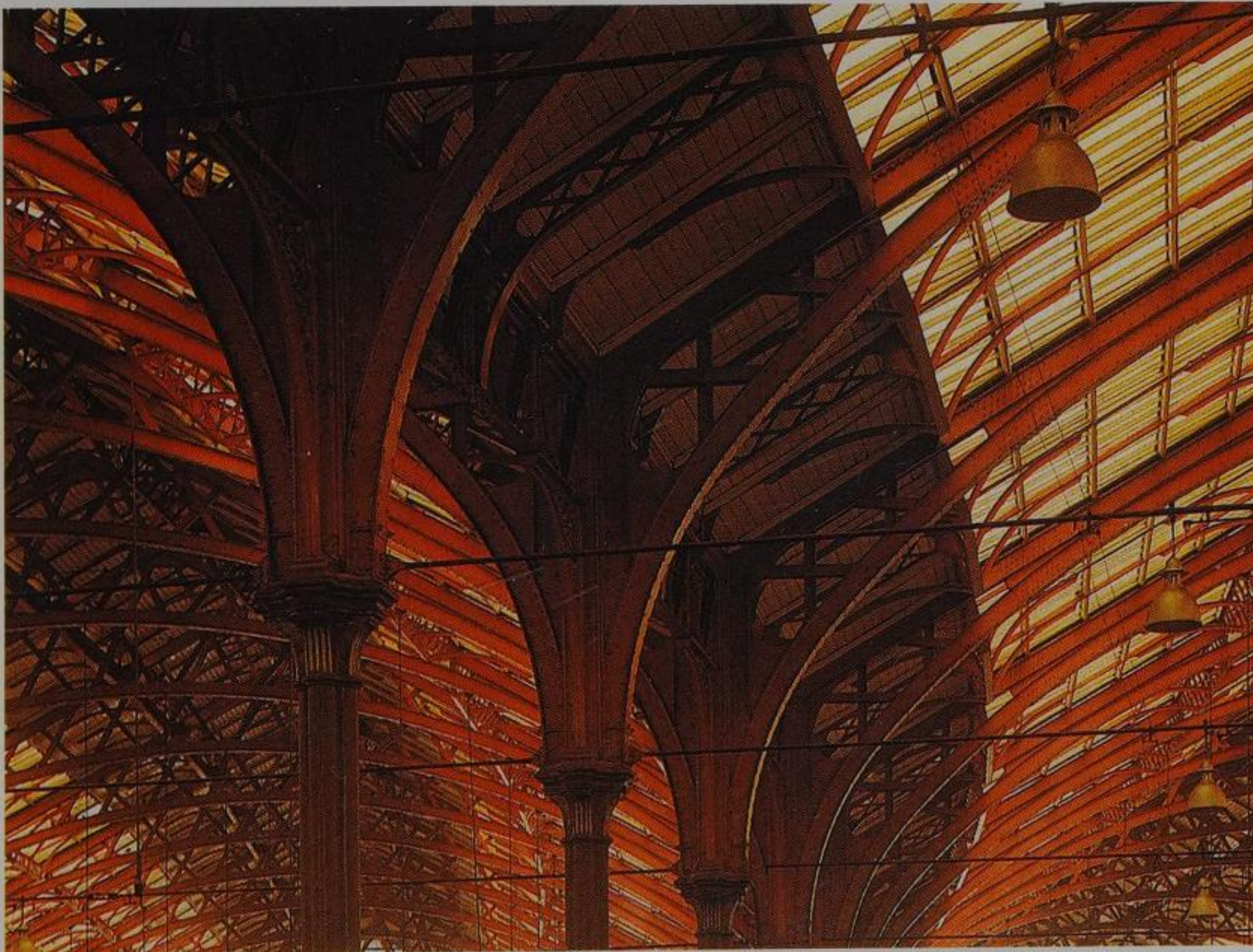
Left: The soaring metal beams and struts of Brighton Station's train shed's roof, installed in 1882 by H E Wallis, attempt to imitate the vertical thrust of Victorian Gothic.
