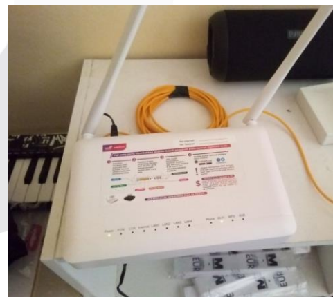
Gambar 6 Optical Network Terminal
