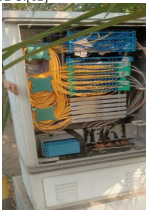
Gambar 4. Optical Distribution Cabinet
