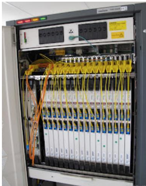
Gambar 2.2 Optical Line Terminal.
