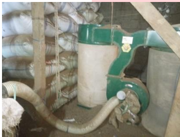
GAMBAR 3 Cyclone Dust Collector Existing
