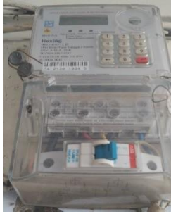
Gambar 2.1 KWH Meter Digital
