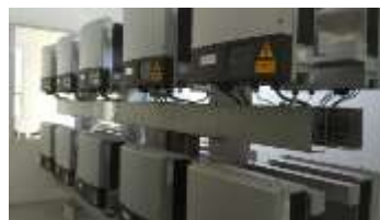
Gambar 3. 9 String Inverter SMA STP5000TL
