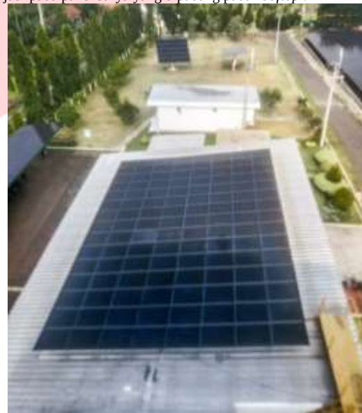
Gambar 4. 7 Rooftop Terkena Shading
