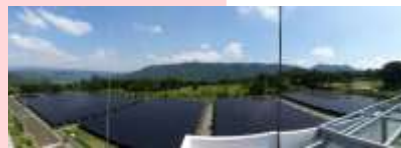
Gambar 3. 5 Array 31 (Ground Mounted)
